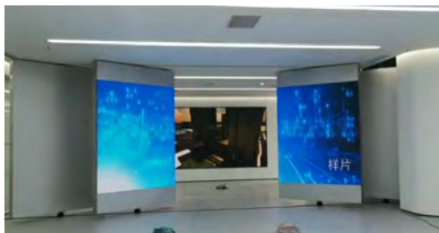
开合屏机械/Opening and closing screen machinery
